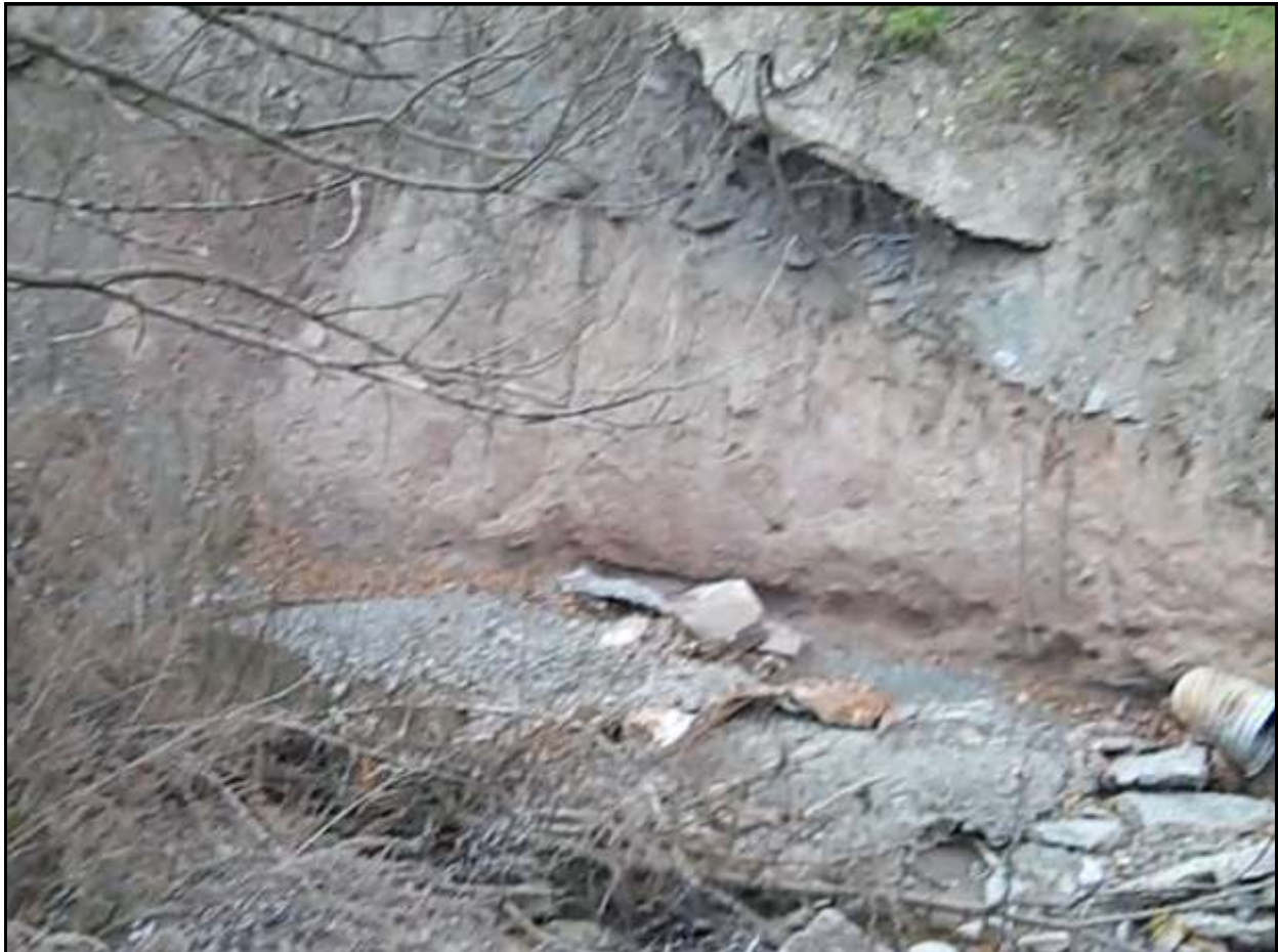
Figure 6: Severe streambank erosion on Hobbie Creek, 200 feet upstream of its confluence with Densmore Creek.
